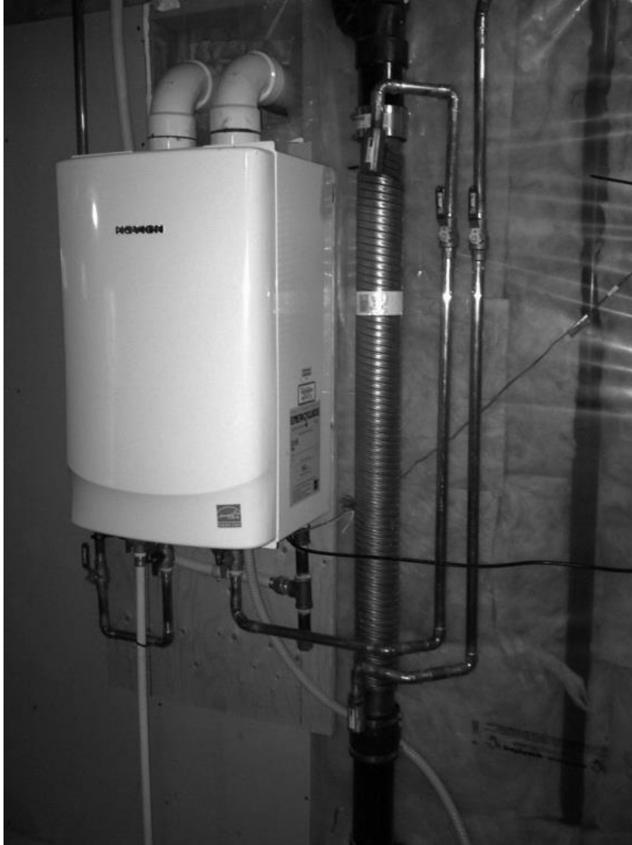
Figure 3-1 A DWHR system connected to a tankless water heater in a basement [23].
