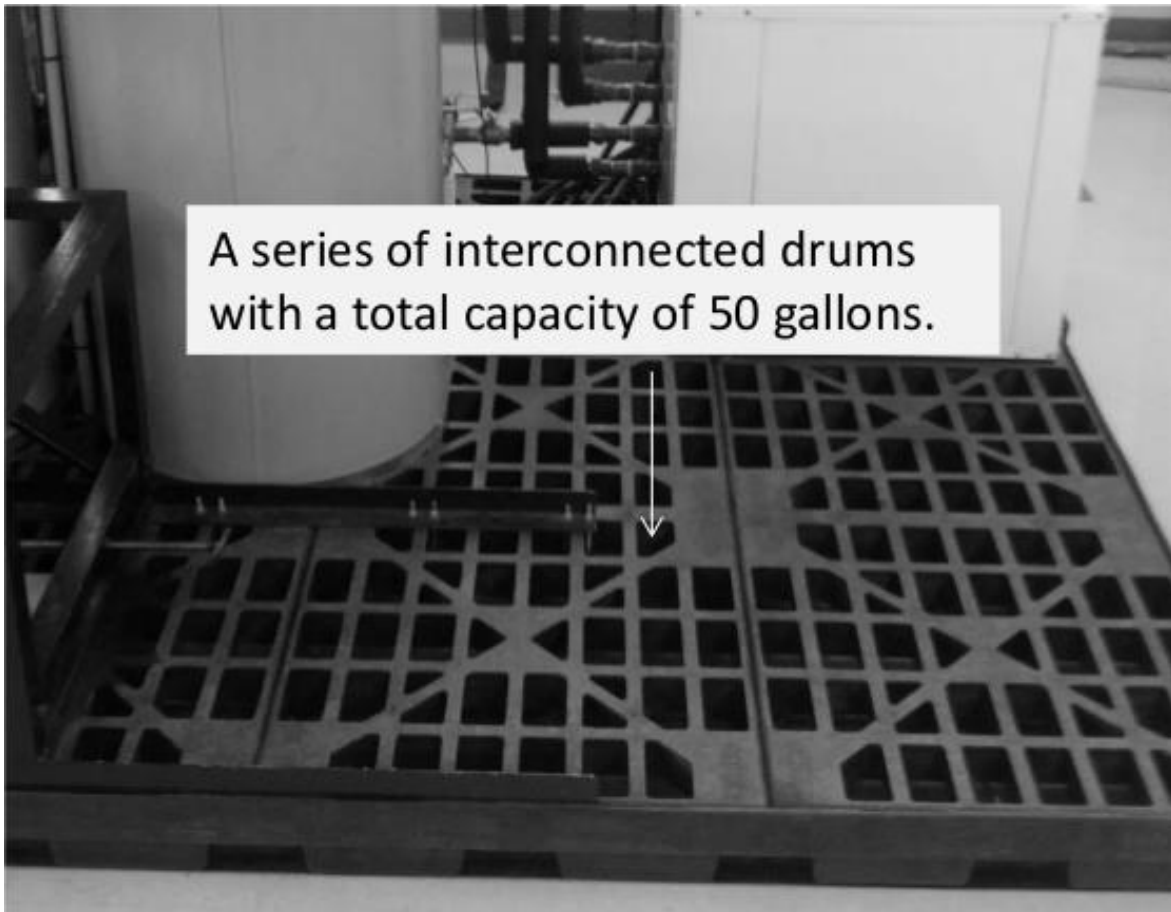
Figure 2-10 Containment platforms installed beneath the test apparatus to prevent water spillage onto the floors.
