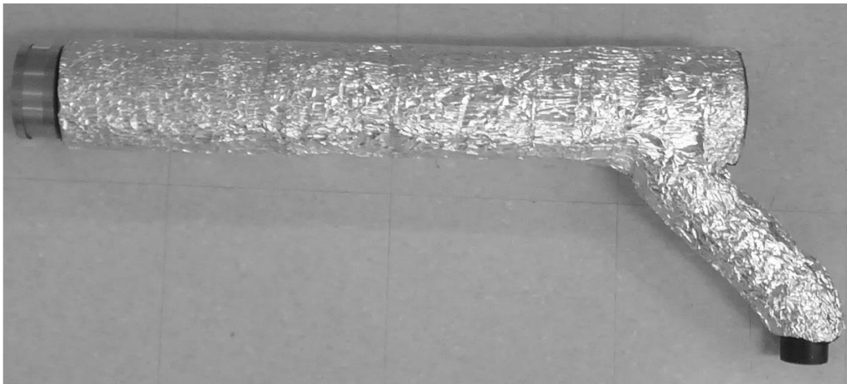
Figure 2-9 The 10.2cm diameter ABS header covered in insulation to minimize thermal losses.
