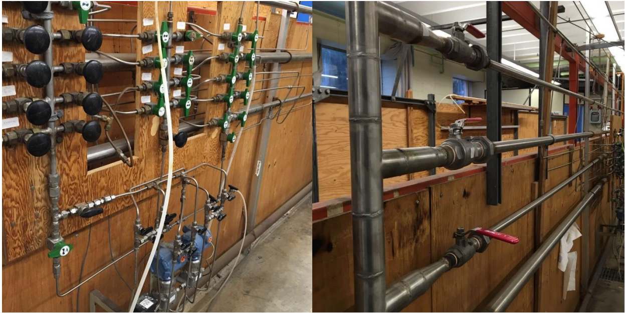
Figure 18 (c) control system and pipeline photo
