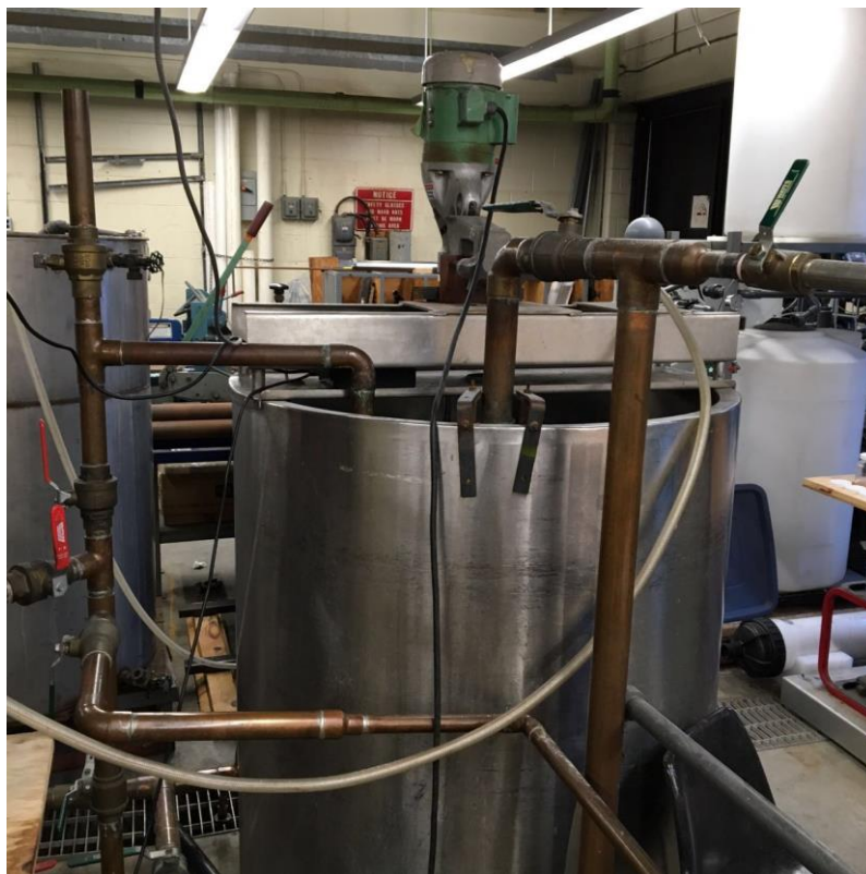
Figure 18 (b) mixing tank photo
