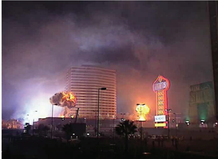
Figure 33: Video stills from the implosion of the Dunes hotel which employed pyrotechnics to dramatize the event (October 22, 1993). Las Vegas Sun
