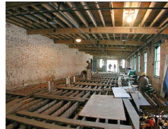
Fig. 1.3.1: Before, Distillery building under renovation to be converted into a restaurant (above)
