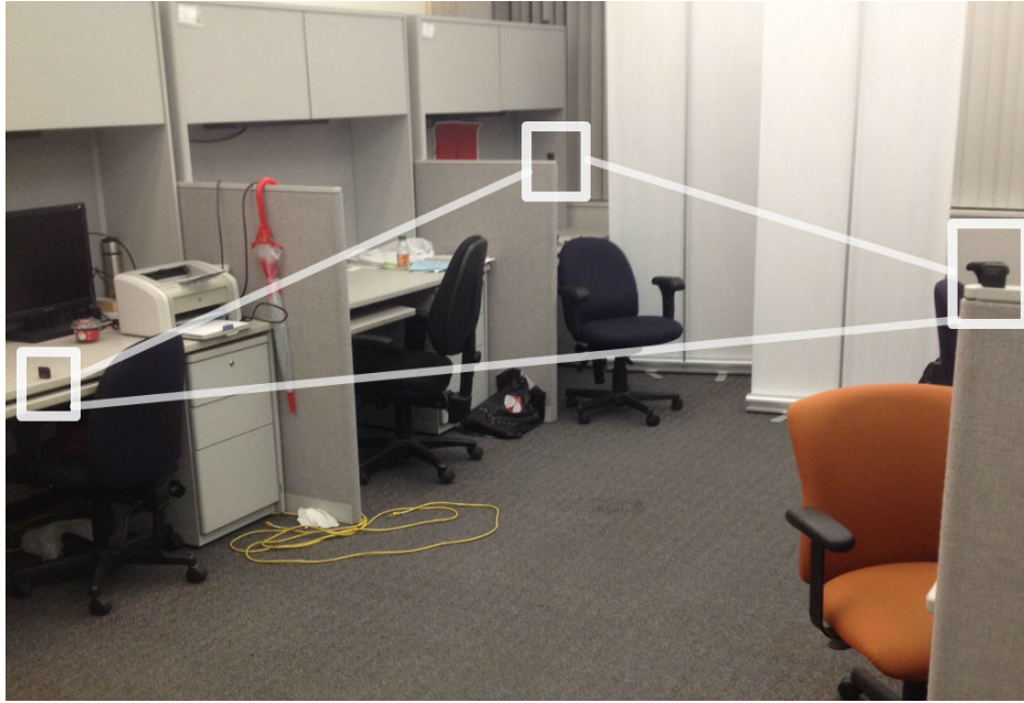
Figure 4.3: The iBeacons in an Office
