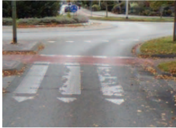
Figure 1.6: Detection Failures from Worn Markings: The marking detection method of [14] fails to detect these markings and flags them for needing maintenance. The detection method of [14] is otherwise very effective for well maintained markings.
