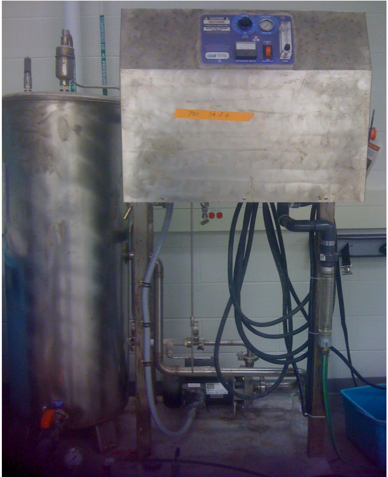
Figure 3.5: Pilot-scale Ozone Generator
