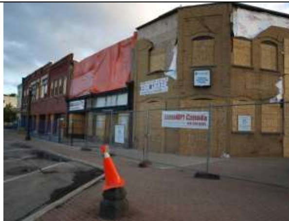
Immediately After Tornado (September 24, 2011)
