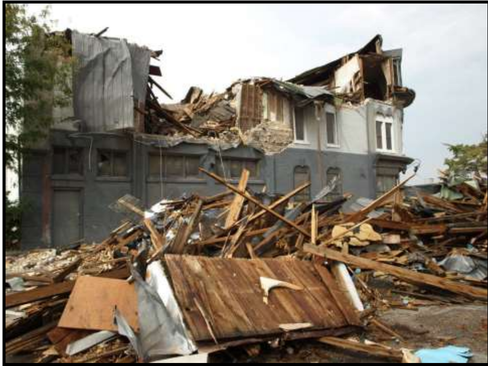
Image 2: Damage to 56-58 Courthouse Square (now demolished) (September 3, 2011)
