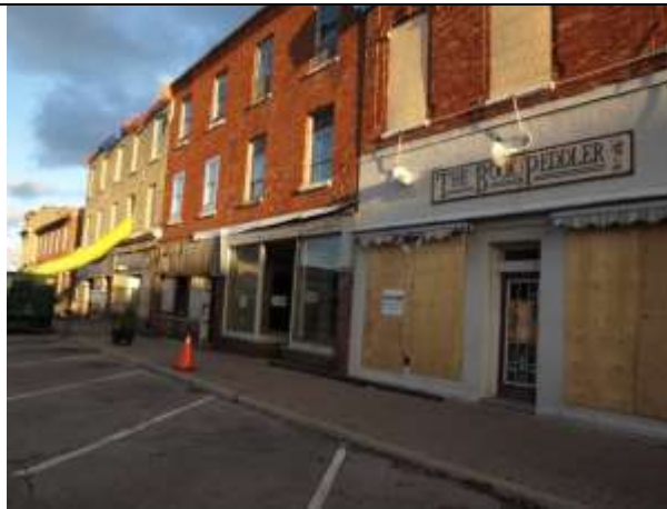
Immediately After Tornado (September 24, 2011)
