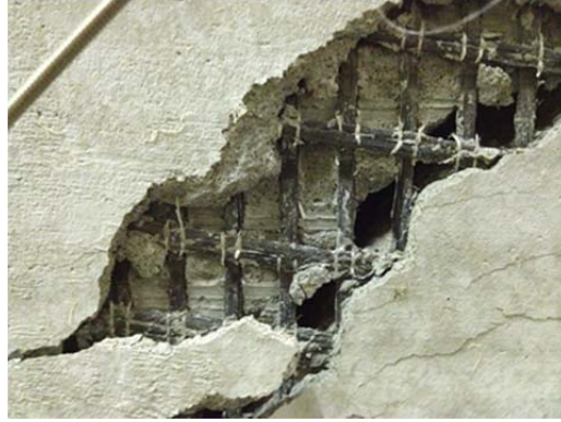
Figure 4.11 : Failure of CFRCM strengthening layer - A closeup view
