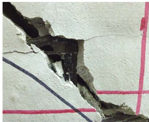
Figure 5.6 : Failure of strengthening layer - A close-up view
