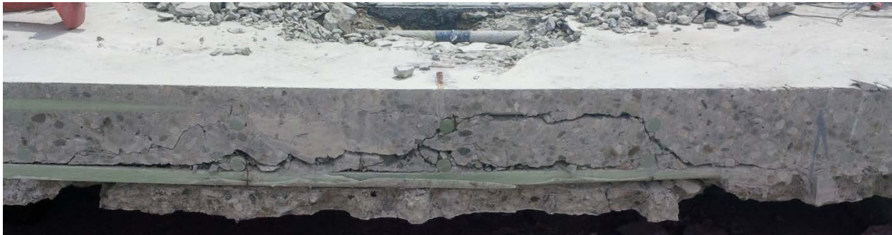
Figure 4-96. SB-1: Punching shear crack near the failure adjacent to the closure strip.
