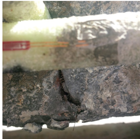
Figure A-34. SB-1: Crack through UHPC.
