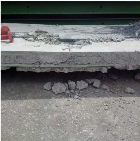
Figure A-31. SB-1: Punch crack seen along cut adjacent to load point adjacent to closure strip.
