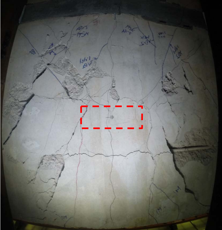
Figure 4-31. SB-3: Underside of slab following failure in centre of precast concrete panel. (Red line indicates load location)
