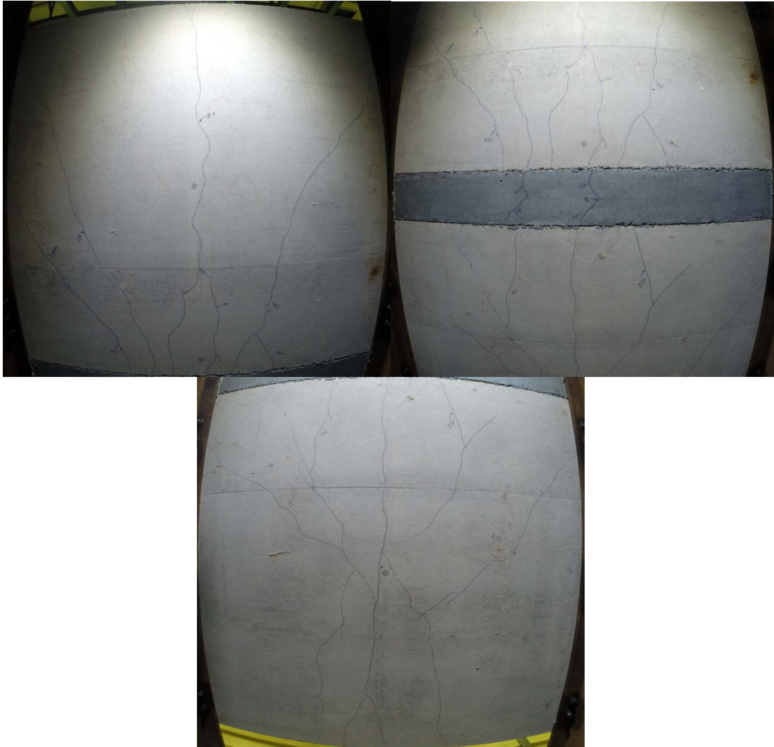
Figure 4-49. SB-1: Underside of slab after fatigue loading. (Top left: slab loaded adjacent to panel, Top Right: closure strip, Bottom: panel loaded in centre)
