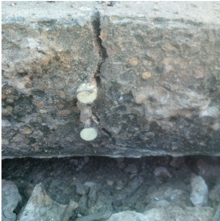
Figure A-38. RB-1: Crack through UHPC (upside-down) at centre longitudinal bar.
