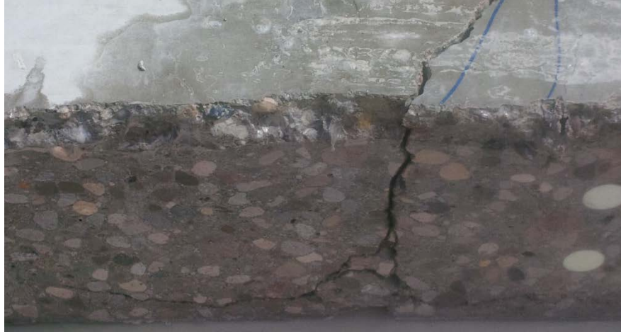
Figure 4-101. RB-1: Crack through the slab, shown by cutting the slab transversely.
