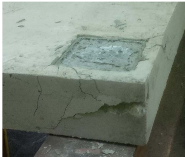
Figure 4-92. RB-1: Concrete cracks near corner shear pocket during failure loading.
