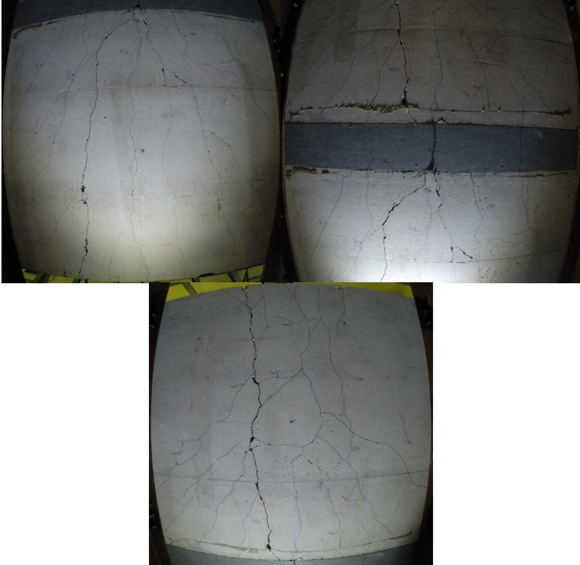
Figure 4-65. RB-3: Underside of slab after fatigue loading. (Top left: slab loaded adjacent to panel, Top Right: closure strip, Bottom: panel loaded in centre)
