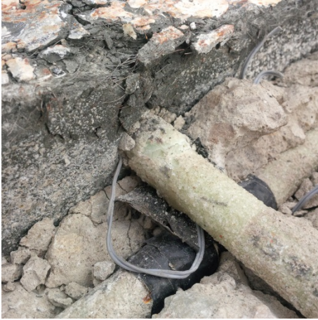
Figure A-1. SB-3: Top longitudinal bar fractured at UHPC interface.
