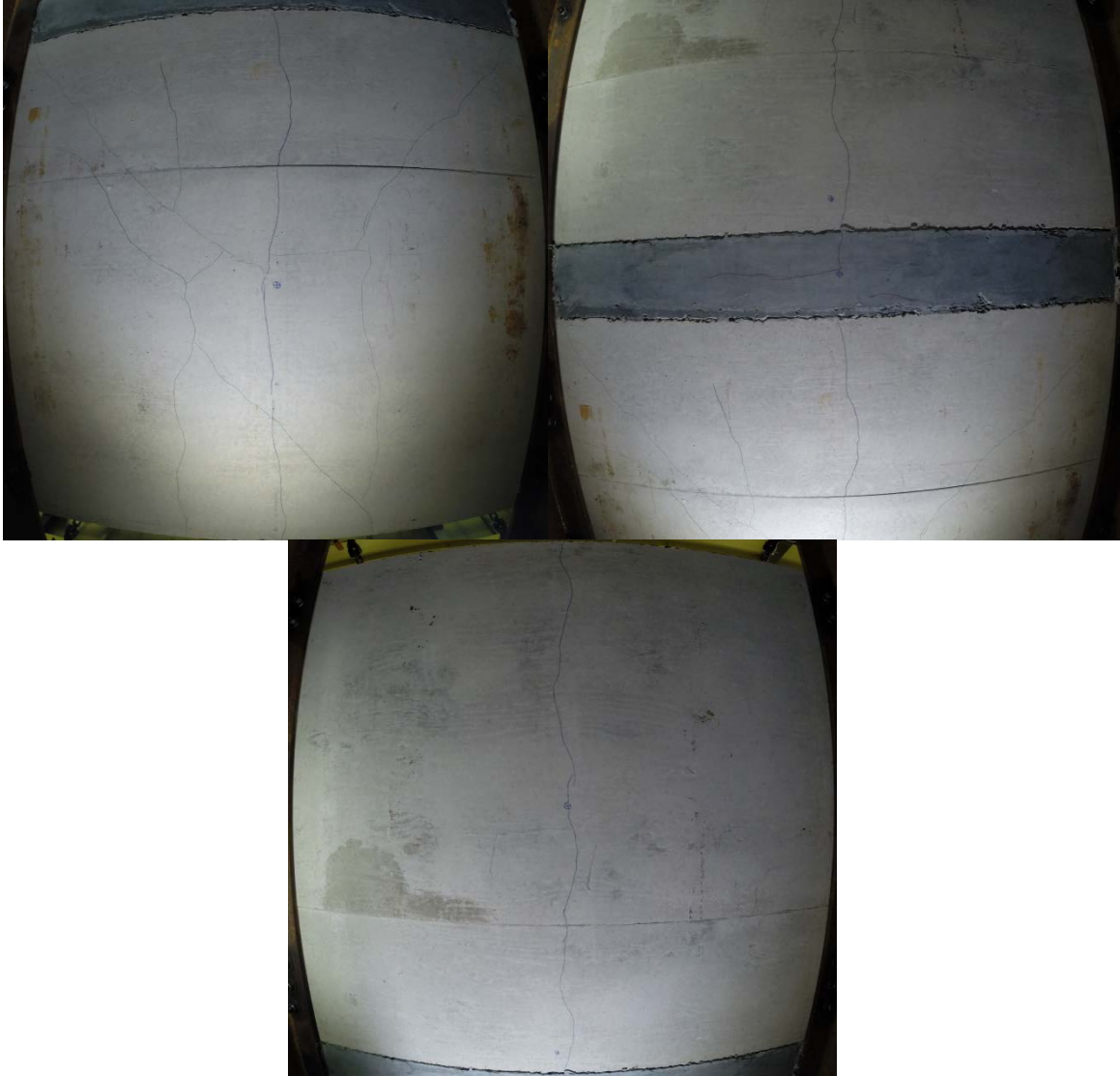
Figure 4-78. RB-1: Underside of slab after initial static loading. (Top left: slab loaded adjacent to panel, Top Right: closure strip, Bottom: panel loaded in centre)
