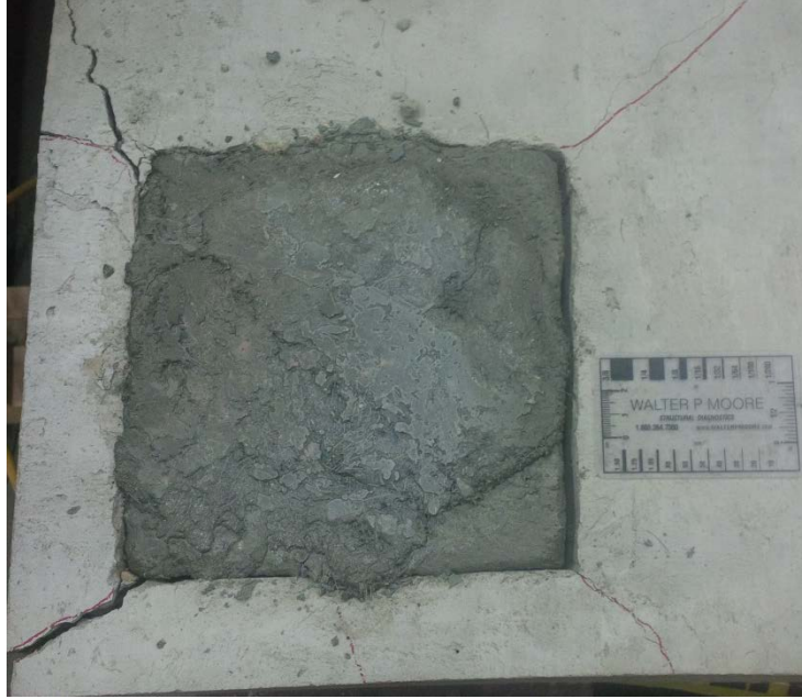
Figure 4-74. RB-3: Cracking and slip of slab near corner shear pocket.
