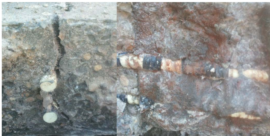
Figure 4-102. RB-1: Crack through the UHPC closure strip as well as the interior of that crack.
