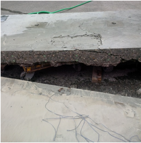
Figure A-30. SB-1: Punch crack seen along section cut adjacent to load point in centre of panel.
