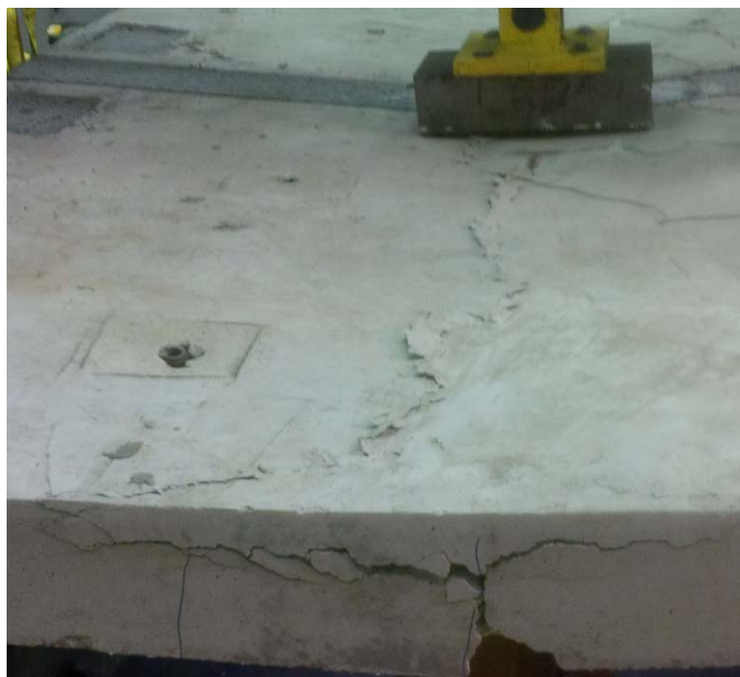
Figure 4-89. RB-1: Concrete crushing on top fibre following failure load.
