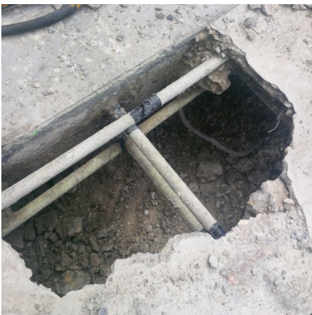
Figure A-32. SB-1: Punch location adjacent to closure strip with concrete removed.
