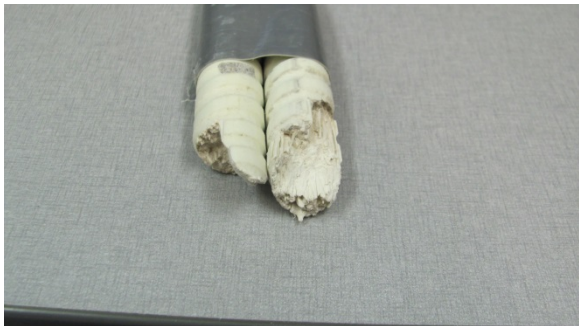
Figure A-22. RB-3: Bottom Bar #9 fracture plane.
