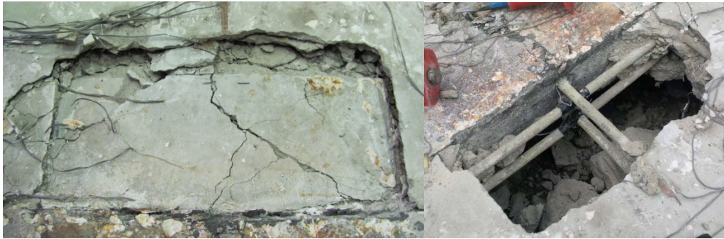
Figure 4-93. SB-3: Top of punched location prior to (left) and after (right) concrete removal.
