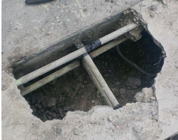
Figure 4-97. SB-1: Punch location with the concrete removed viewed from top of slab.
