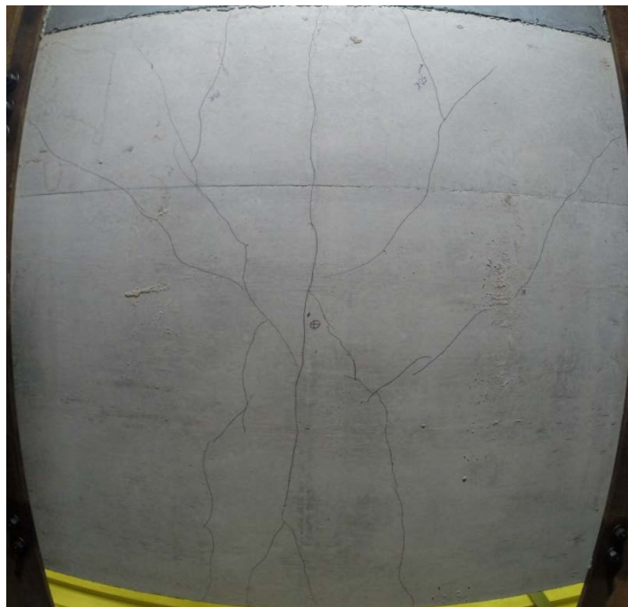
Figure 4-36. SB-1: Crack pattern on precast panel after initial static loads.
