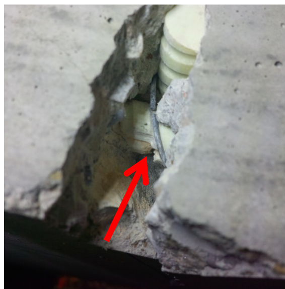
Figure 4-62. RB-3: Broken transverse bar at edge of slab. Arrow indicates fracture location.
