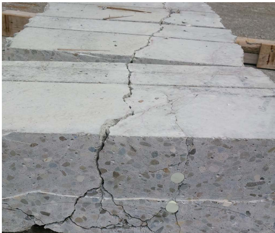
Figure 4-99. RB-3: Crack through the underside (shown up) of the slab and seen through a transverse cut through the slab.
