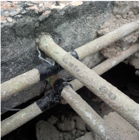
Figure A-2. SB-3: Reinforcement after removal of the punched concrete cone.
