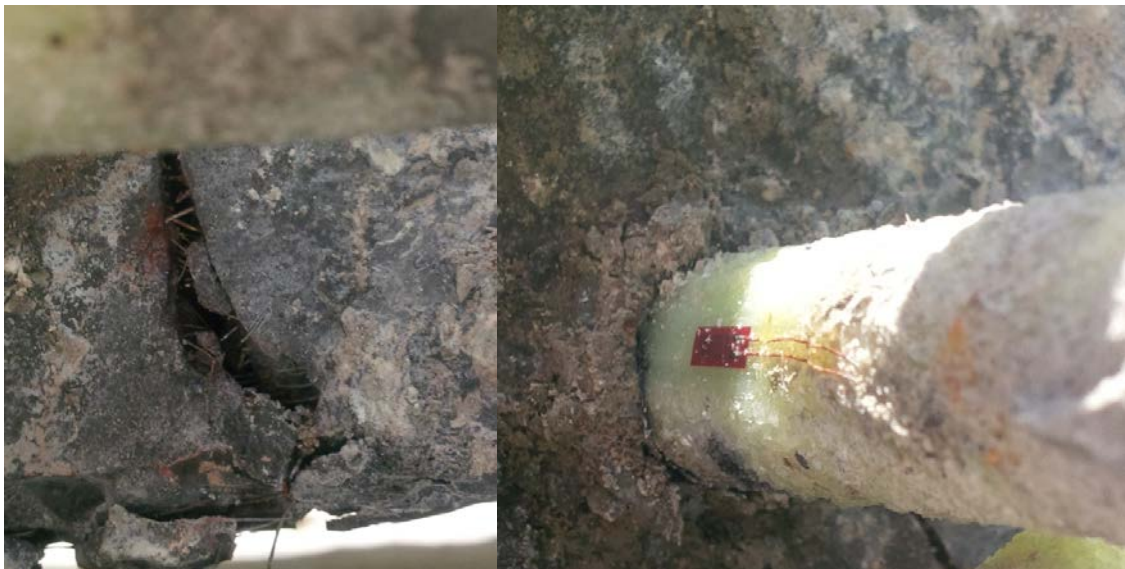
Figure 4-98. SB-1: Crack through the UHPC and longitudinal bar embedded in the UHPC.
