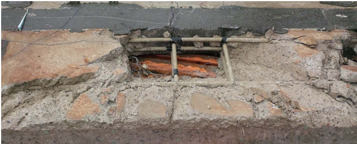
Figure 4-95. SB-3: Underside of panel after failure adjacent to the panel with concrete removed.
