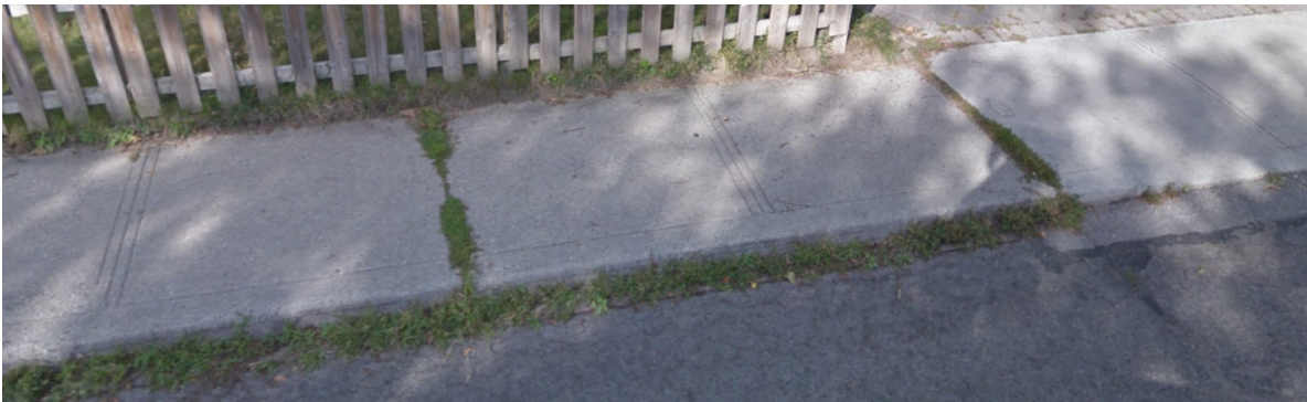
Figure 23: Tripping Hazard on Segment W24, Highview Crescent (Lee, 2016)
