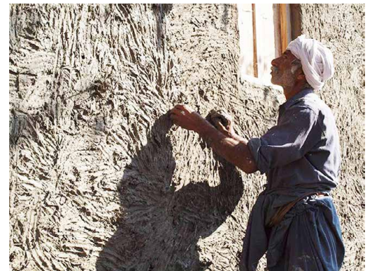
Figure 4.8: Local materials are often chosen in humanitarian efforts, such as the Earth Home Project which helped villagers in Pakistan rebuild homes after a flood.
