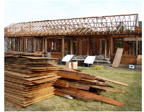
Figure 6.8: "Business as usual" demolition, material sorting on-site, deconstruction and stockpiling of materials.
