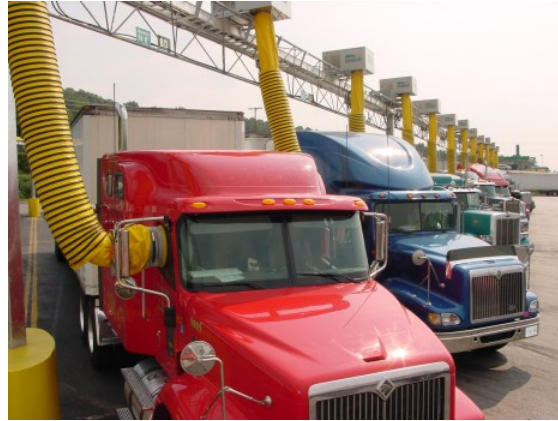
Figure 2.4 Advanced Travel Center Electrification services by IdleAir [29]
