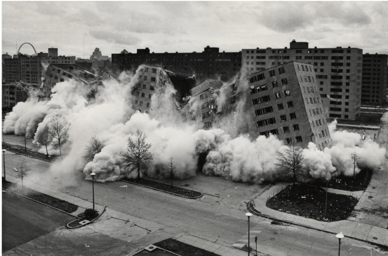
Figure 2.20- Still image from Pruitt-Igoe's first demolition on March 16, 1972. The demolition footage was widely televised and also incorporated into the 1982 experimental film 'Koyaanisqatsi' directed by Godfrey Reggio which has achieved cult status since its premiere.
