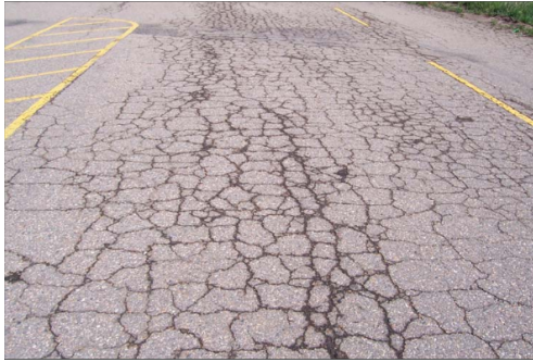
(a) Severe alligator cracks [2]
