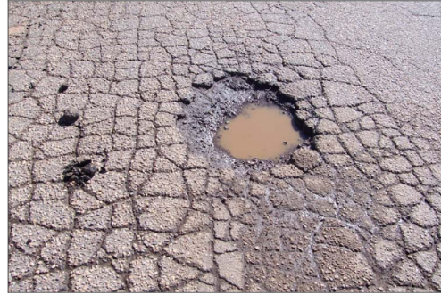
(d) Large pothole surrounded by alligator cracks [2]
