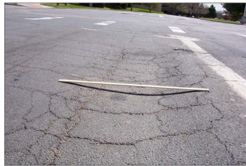
(f) Severe rutting [2]
