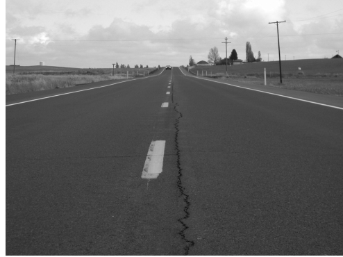
(b) Severe longitudinal crack [34]
