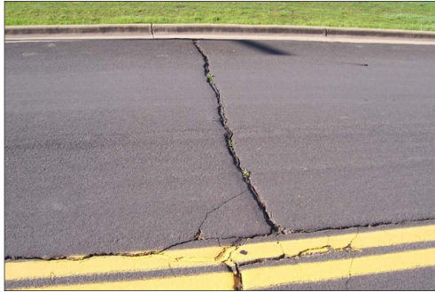
(c) Severe transverse crack [2]
