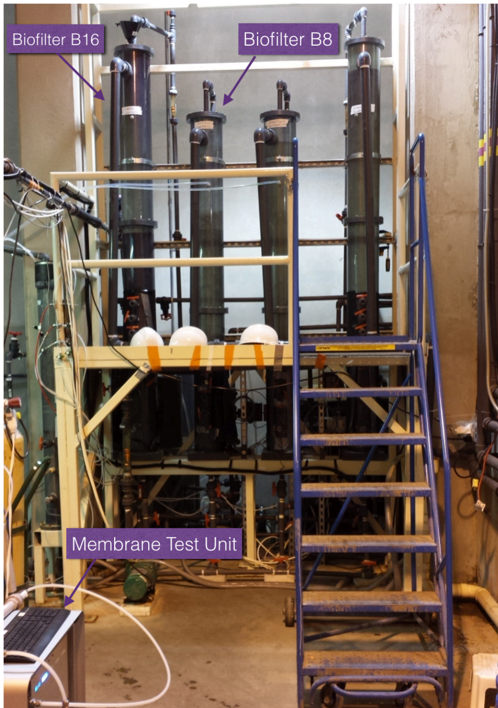
Figure A-5 – Biofiltration pilot plant set up at the Mannheim Water Treatment plant in Kitchener, Waterloo, Ontario.
