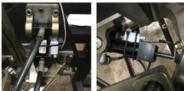
Figure 6-19: Linear potentiometers installed on the actuators to provide feedback on the length of the actuators.
