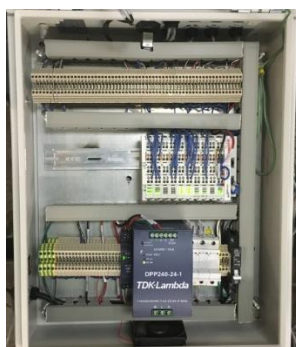
Figure 6-18: Beckhoff control panel.
