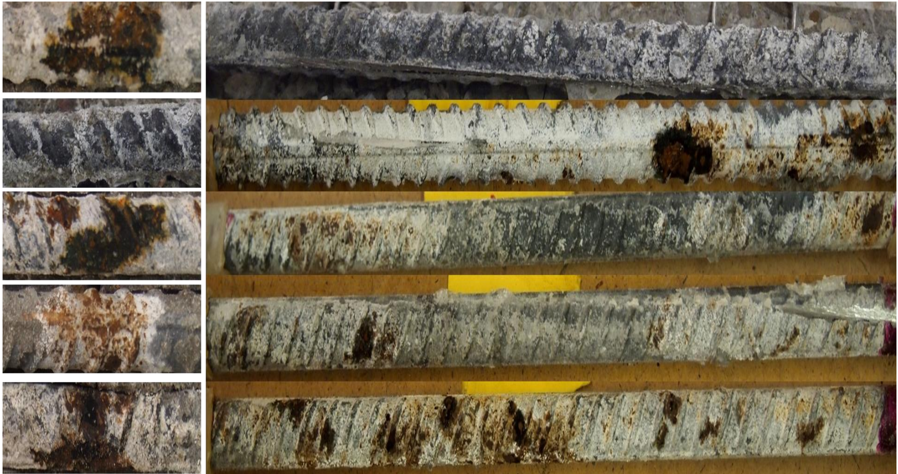
Figure E2.3.1: Exposed surface (to concrete crack) of transversely- (left) and longitudinally- (right) cracked C3 steel specimen 1 to 5.
