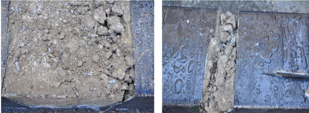
Figure 4.3 Mode of failure for wrapped beam
