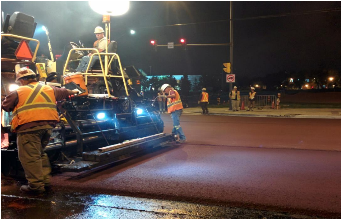
Figure 3-5 Red Asphalt Paving on a Section of Highway 7 BRT Lane York Region ON, August 21 st 2014
