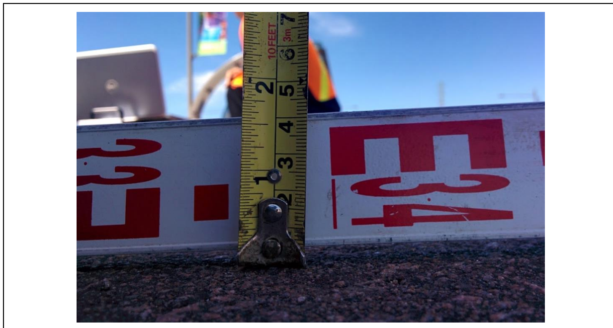
Figure 5-5 Close-up View of Rutting Depth of a Section on Highway 7 BRT-lane May 2016, York Region, ON
