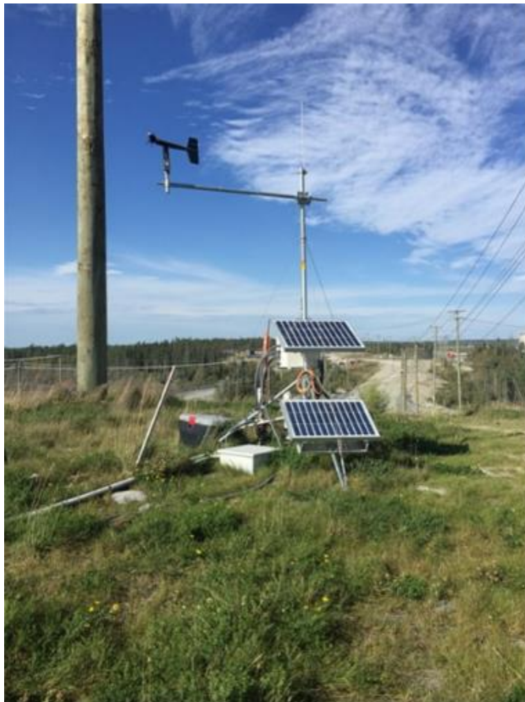
Figure 2-5 – Instrumentation on WRS#3 used to record and log pressure and gas-concentration data
