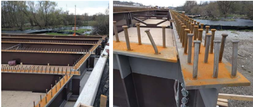
Figure 2-1: Exposed headed studs prior to the casting of the CIP concrete deck.
