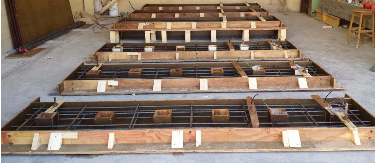
Figure 3-11: The precast formwork laid flat on the ground, while the CIP formwork was shored.
