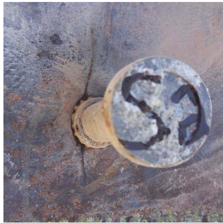
Figure 4-20: Fatigue crack propagating transversely through top flange at S2 in Specimen P200.
