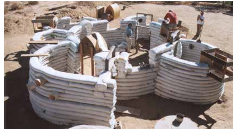
Fig 3.08 SuperAdobe is an earth bag architecture developed by the Iranian architect Nader Khalili. This building system needs long sandbags, barbed wire, on-site earth, and a few tools. One of the biggest advantages of this system is that it has passed severe earthquake code tests in California. 38 However, it should be noted that this structure is more permanent than temporary and building it would require dealing with land rights, construction permissions and etc. Moreover, the dimensions and the permanency of this design proposal is a major drawback in post disaster cases where the affected families would like to have their temporary houses next to their damaged property.
