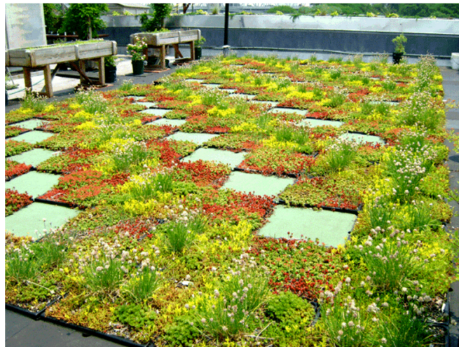
Figure 3.5 Green Roof with Wildflowers, New York (greenroofs.com, 2016)
