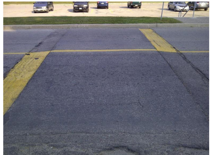
Figure 18. Image of the bump over which vehicle was tested
