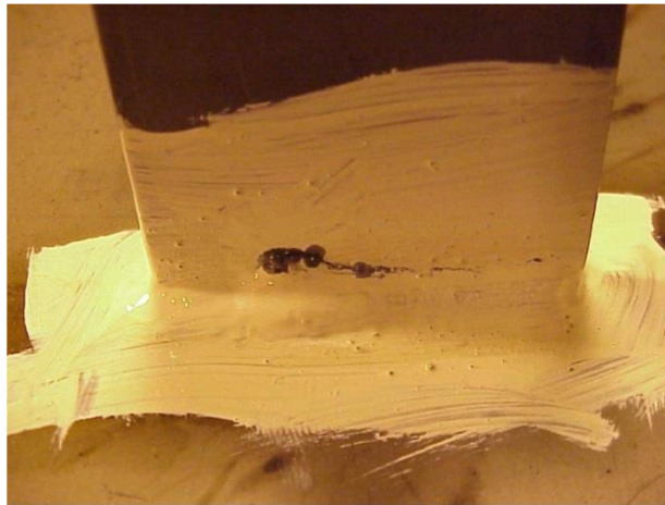
Figure A1- 30: Crack location in the attachment plate’s upper weld toe of the T-joint subjected to out-of-plane cyclic loading
