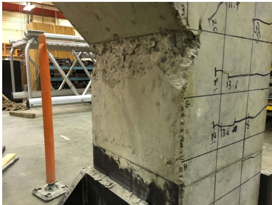
Figure A.30: Extent of Crushing, UB-3-6
