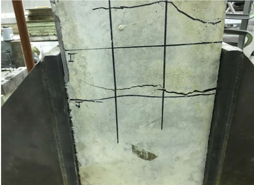
Figure A.36: Wide Crack in Column Base Causing Debonding. CA-2-6
