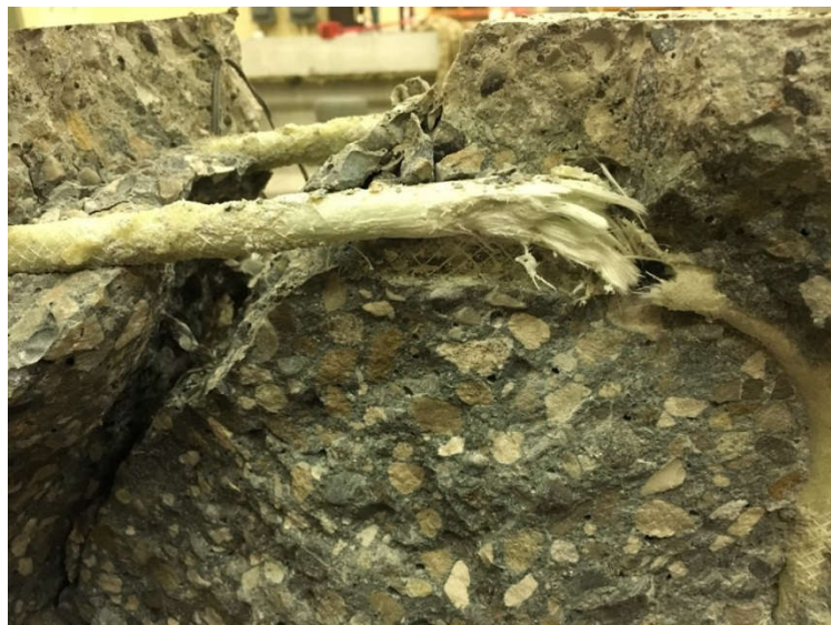
Figure A.50: Closeup of Bar Rupture, UA-2-4
