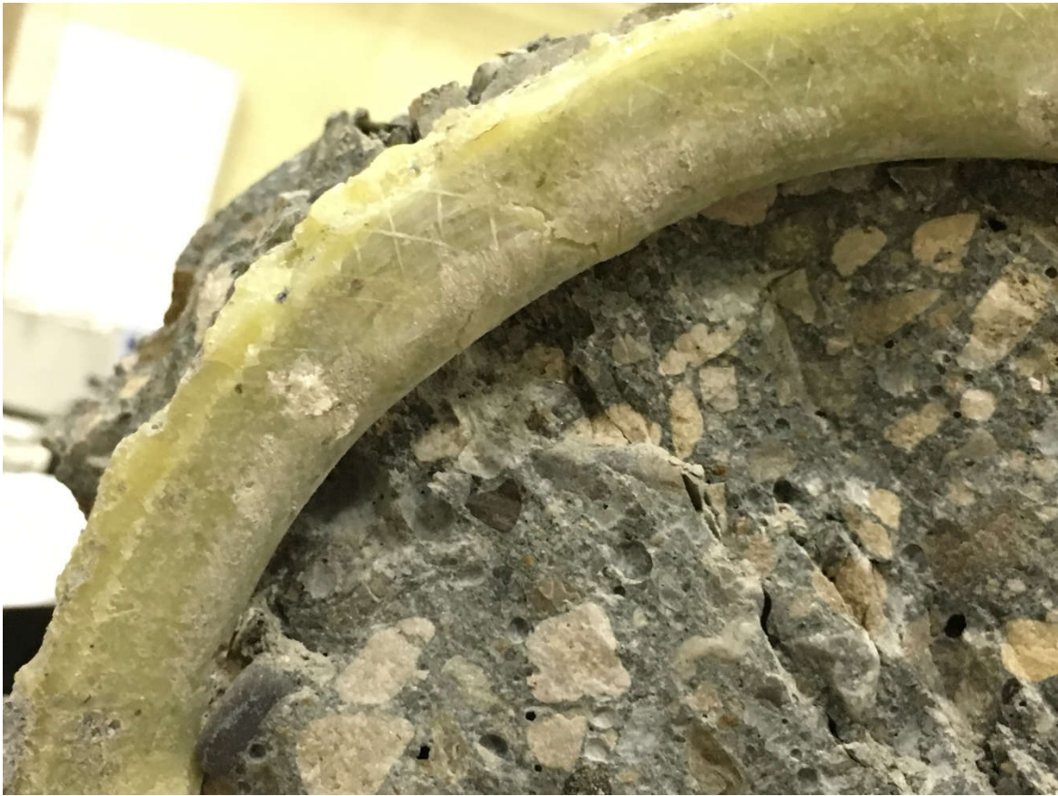
Figure A.22: Crack in Bend, UA-3-6
