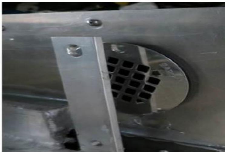
Figure 74: Battery Pack Vent
