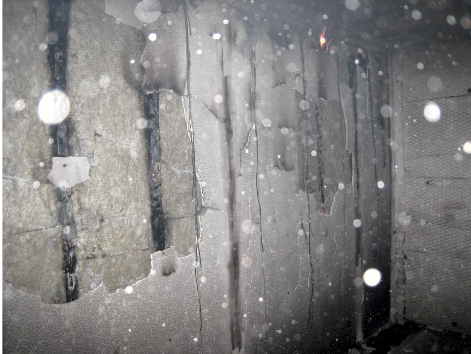
Figure 3.16: State of the wall post-fire ( t = 45 min).
