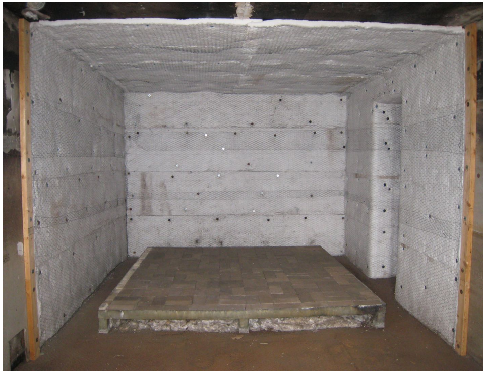
Figure 3.3: Fire compartment with ceramic fibre insulation interior lining.
