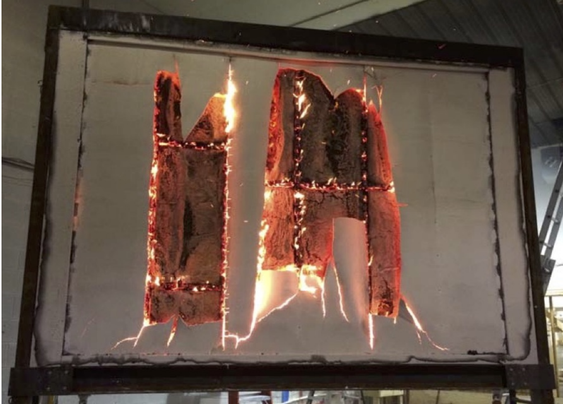
Figure 7.54: Condition of the EW1 wall in the furnace test after 60 min of exposure.
