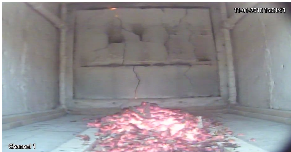
Figure 7.36: Real wall test #4, fire-side camera, 55.6 min.
