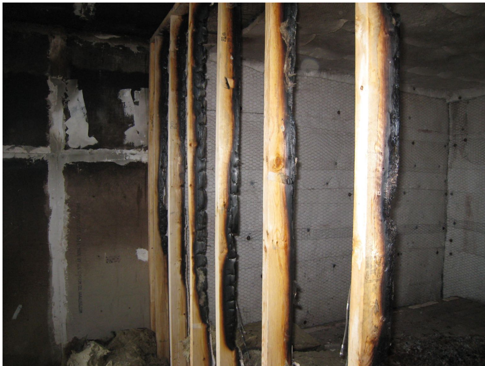
Figure 3.17: Depths of charring of the wood studs.
