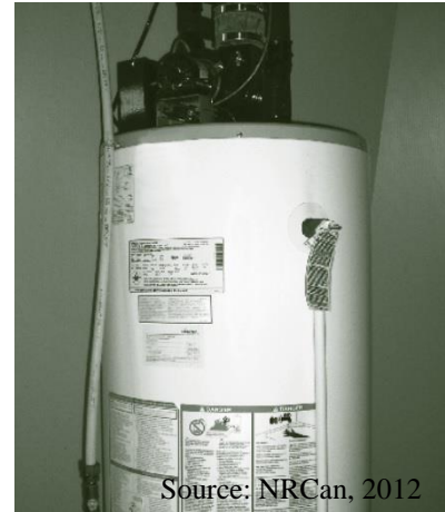
Figure 55: Power Vented Gas Fired Water Heater
