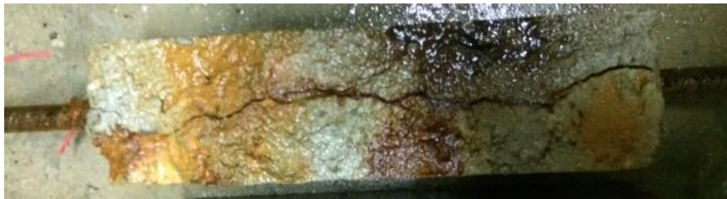
Figure 5.5 Corrosion-induced cracking of the concrete prism
