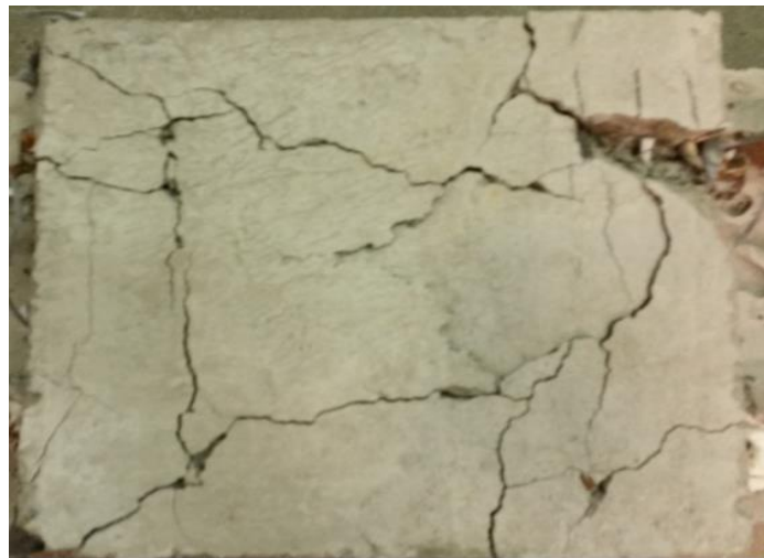
Figure 6.3 Bottom face cracks of beam confined with internal transverse reinforcement
