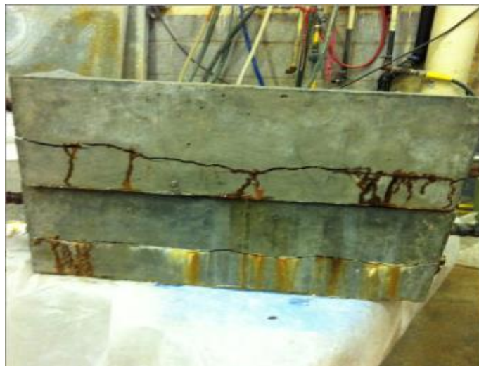
Figure 3.6 Corrosion pattern of the rebar in a concrete prism
