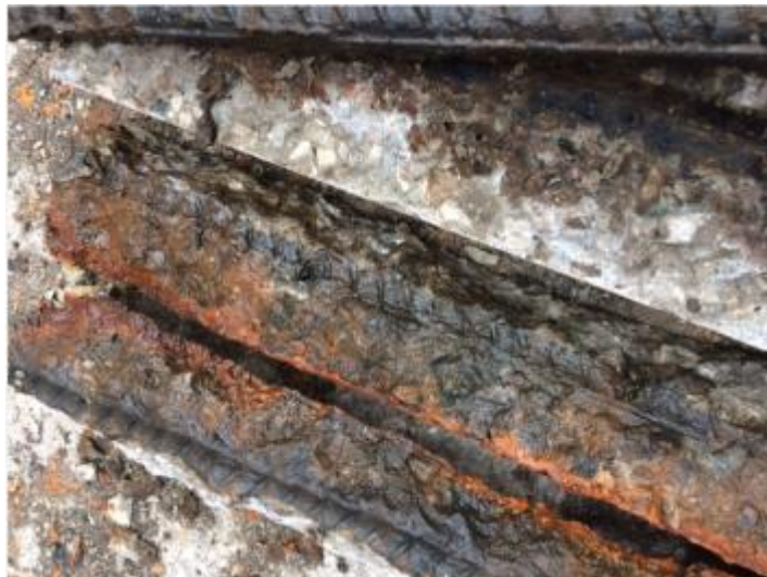
Figure 5.6 Corrosion products at the interface between the rebar and the concrete
