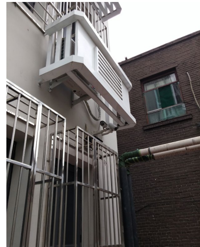
Fig 1.25. Window Guards in an Elementary School
