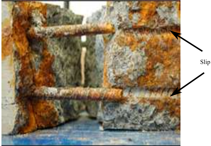
Figure 1.2: Loss of bonding between concrete and the embedded steel bars, resulting in slip [2]
