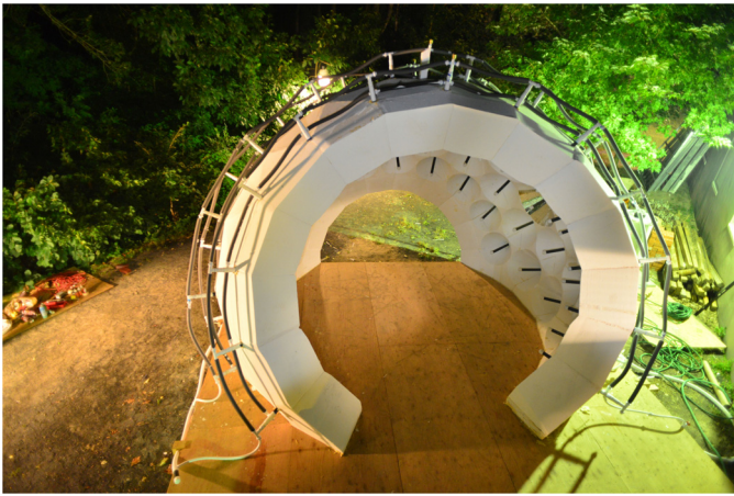
Fig. 1. The Thermoheliodome just after the construction of structure and system was completed in 2014, where the dome's arch follows the sun path on the summer solstice, and the cones will be lined with mylar to reflect radiation onto the coaxial pipes for radiant cooling.
