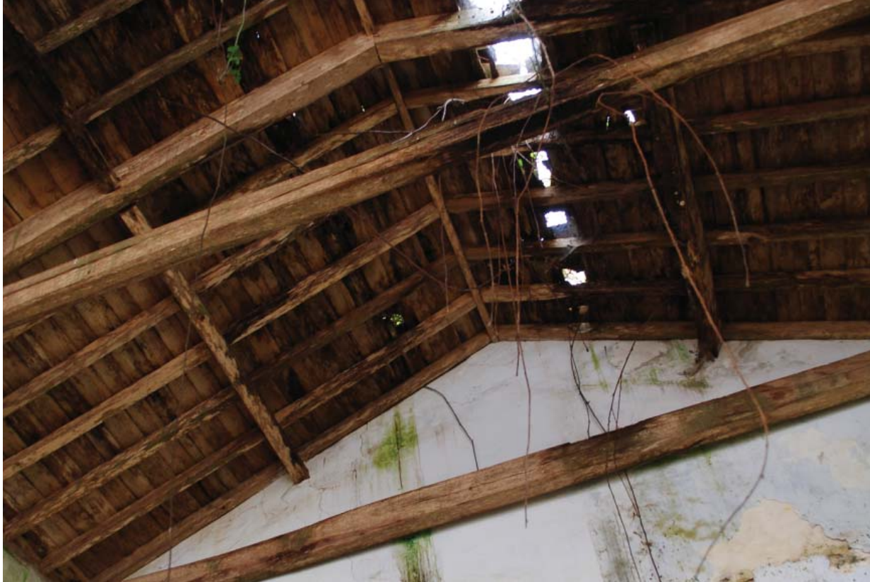
Fig. 1.70. Wooden roof structure in the abandoned chapel of the “Casa da Salga”
