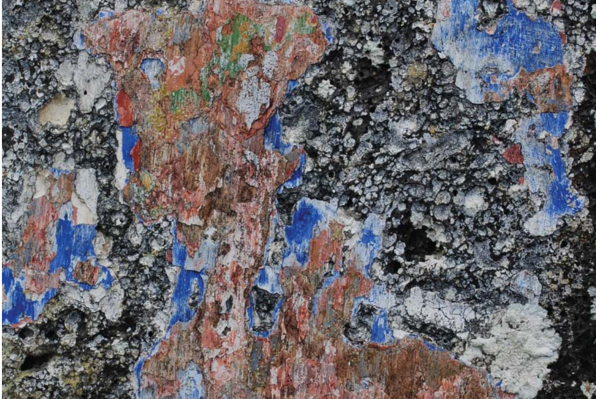
Fig. 1.74. Paint layers on the window frame of abandoned house
