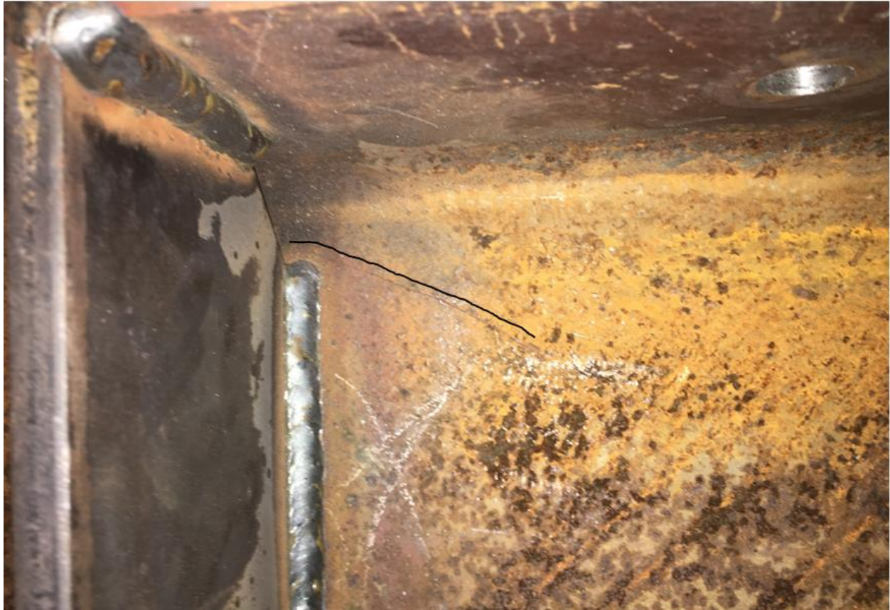
Figure 4–16: Fatigue crack in the web of the steel girder at the West end of Specimen B1
