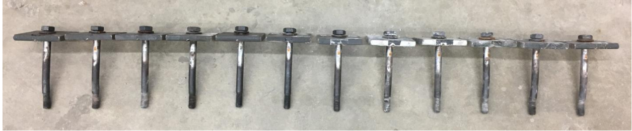
Figure 4–33: Specimen B2 through-bolts S1 - N12 (Left to Right)
