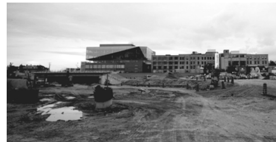
Fig 117. Bottom right. Road construction of the area surrounding the rail underpass at King and Victoria Streets near the future transit hub site in Downtown Kitchener, with Google Headquarters in the background.
