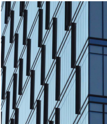
FIG. 2 FACADE AFTER RESKINNING Image of the facade replaced with the glass curtain/window wall systems showing the randomized fins and narrow mullion spacing, mimicking the grille.
