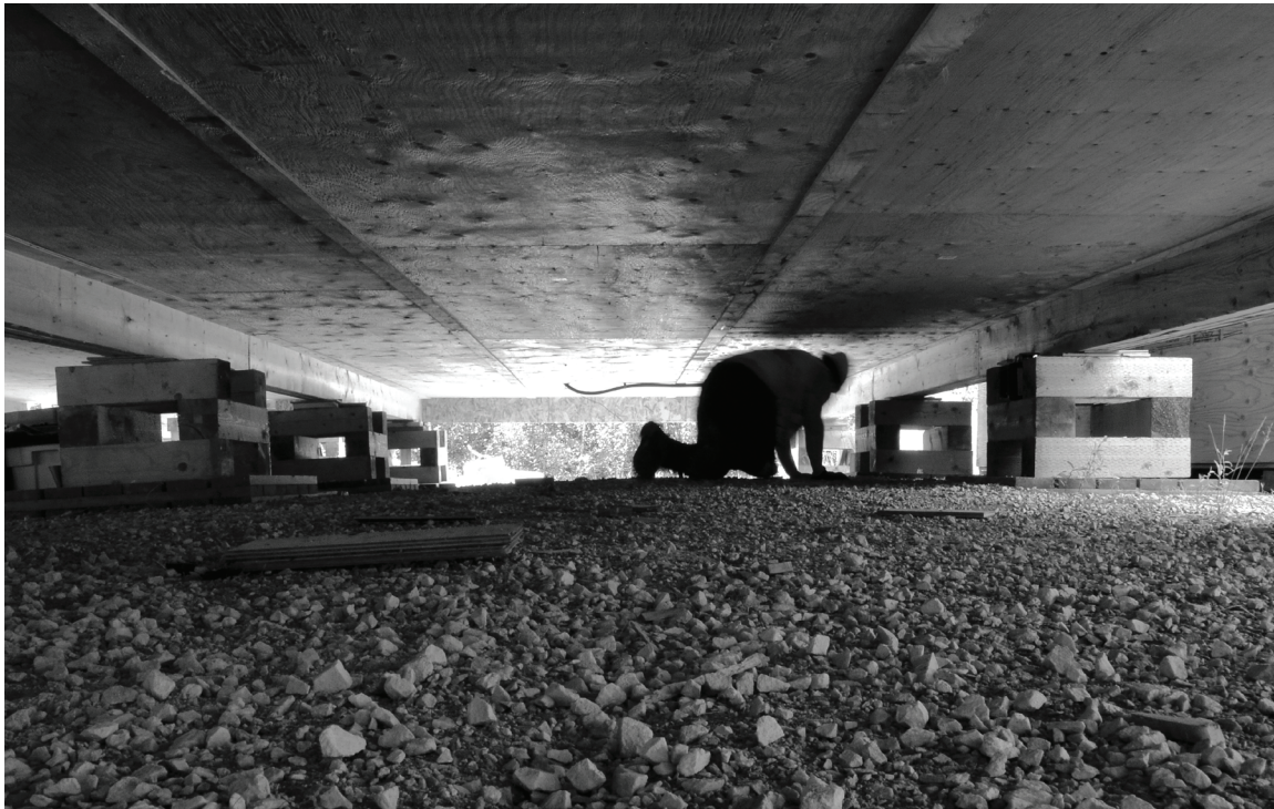
fig. 4.2 Knowledgeable builders work to level the foundations beneath a house. The building sits on a gravel pad that can shift.
