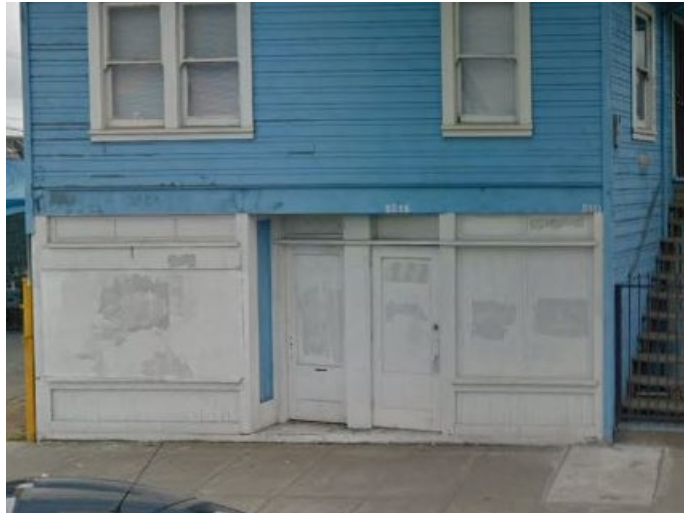
Fig. 1.39 Boarded ground floor, International Blvd.
