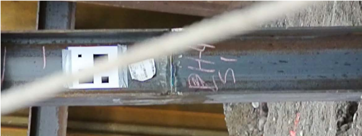
Figure 35 – Pile H-1 with Rope Interfering with Processing of the Image
