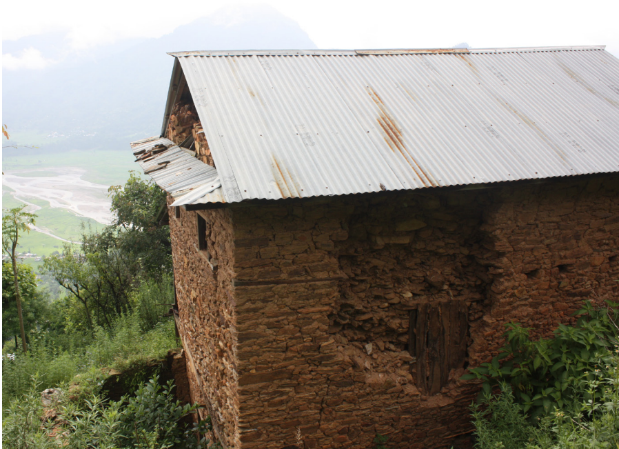
fig. 2.38 Layers of stones make up the thick walls, however with mud as mortar and no reinforcement they are easily damaged under earthquake loading
