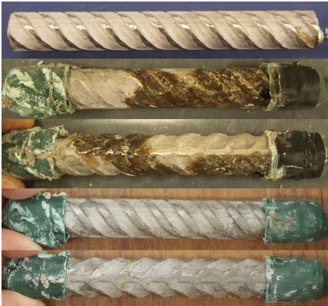
Figure 4.12: RST 4-400 Batch – Corrosion Products on XM-28 AR 7.7. From top to bottom, a) original specimen, b) corrosion products on specimen upon removal from concrete, and c) pitting corrosion identification on a pickled specimen. Slight staining at the top of the bar from the soldering process was observed prior to casting the bar in concrete.
