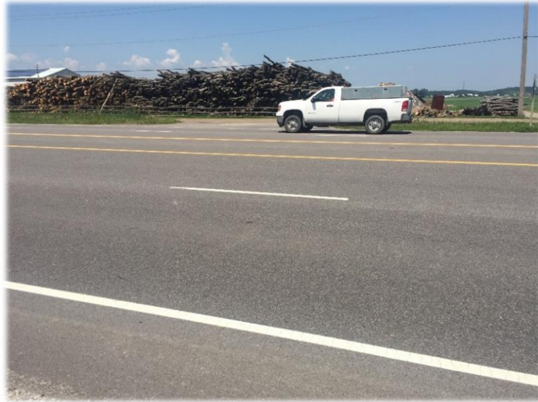
Figure 3-21: Condition of Highway 9, Three Years after Construction
