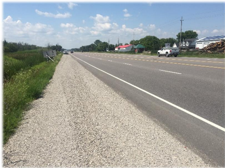
Figure 3-22: Condition of Highway 9, Three Years after Construction
