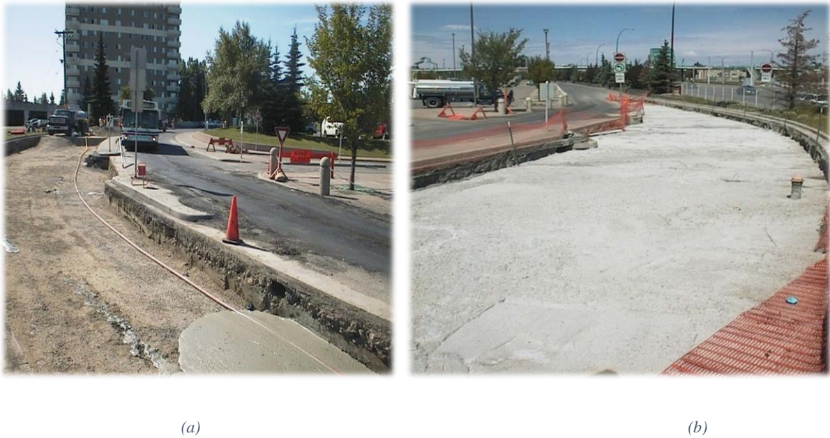
Figure 3-12: Bus Lane. (a) Reconstruction Process. Placing the LCC (CEMATRIX) (b) After Installing the LCC Layer (CEMATRIX)
