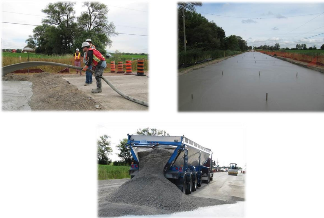
Figure 3-4: Construction Process of Dixie Road, Region of Peel, Caledon, Ontario, Canada (CEMATRIX)
