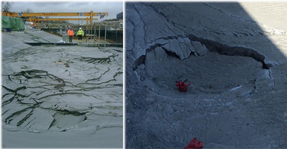
Figure 2-4: Instability Issues with Ultra-Low Density LCC (Field Performance)
