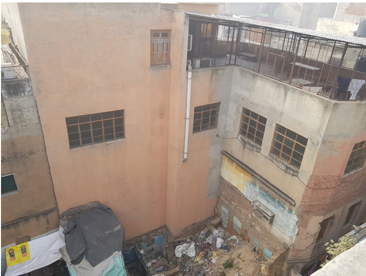
Figure 4.14 One of the collapsed building appears to have been 3 storey high
