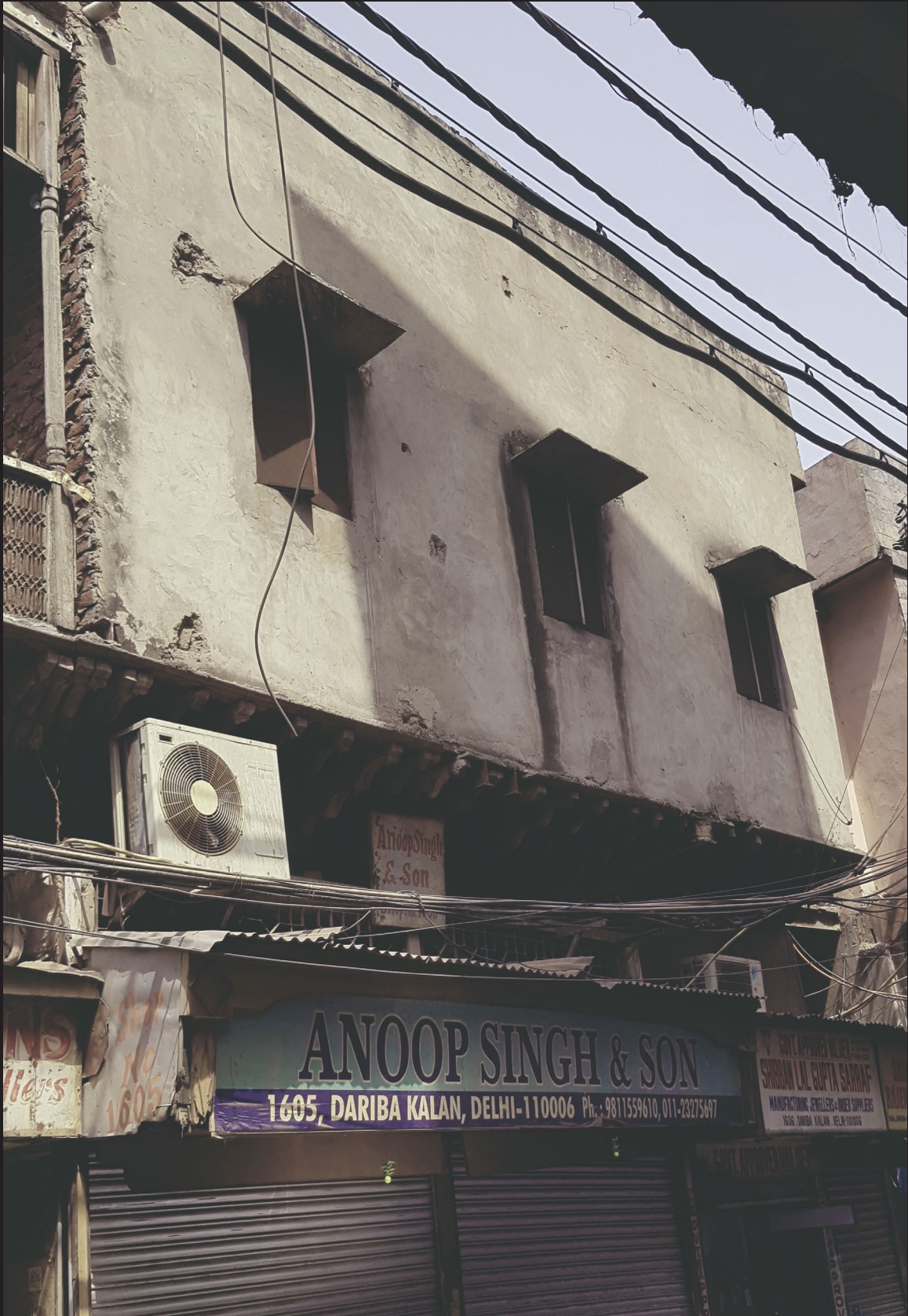
Figure 5.04 Jharokha (enclosed balcony) converted into a room cantilevered on wooden supports.
