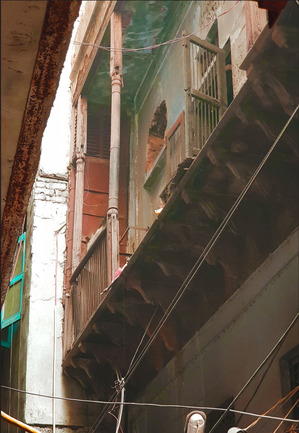
Figure 5.05 Abandoned house - dangerously dilapidated. Vulnerable to heavy rains during seasonal monsoon down pour.
