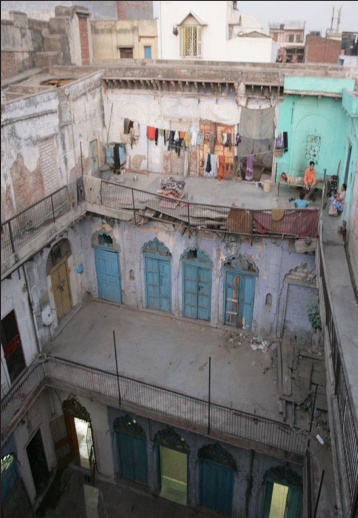
Figure 6.09 Mansion Dharampura - Dilapidated Condition
