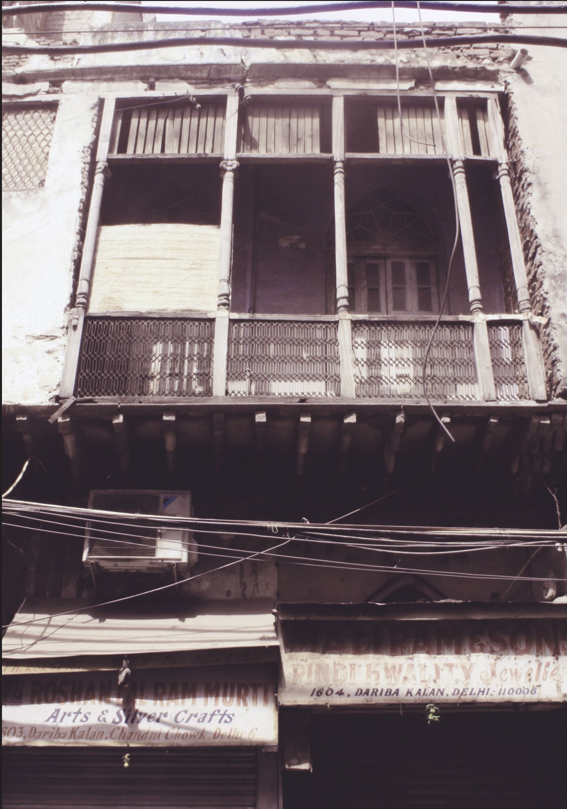
Figure 5.01 Decrepit Condition of housing - Wooden supports, railing and planks used for the Jharokha (enclosed balcony)
