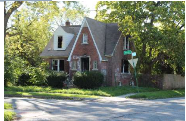
Figure 1.4: Fire Damaged Structures. Photo Montage by Author
