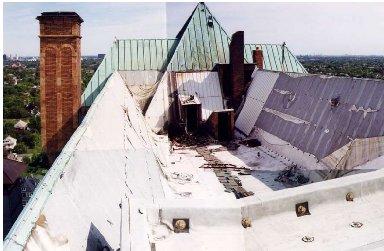
Figure 3.22. Copper roof stripped by scrappers at Lee Plaza Hotel Roof. Source: Scott Hocking, Scrappers , Oswalt, Shrinking Cities: International Research (2005), Pg. 478
