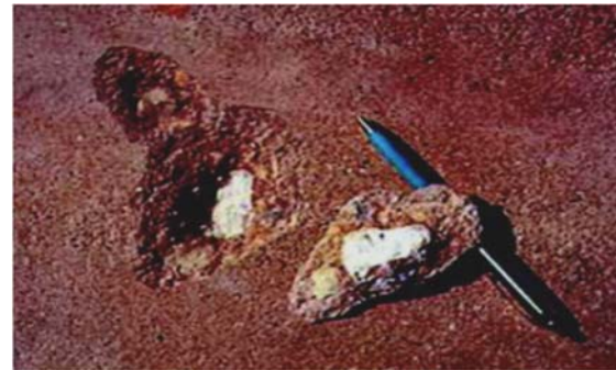
Figure 2-6: Concrete surface with medium popout (ACI 201.1R-08)
