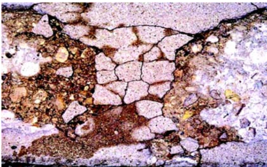
Figure 2-7: Concrete surface with severe scaling (ACI 201.1R-08)
