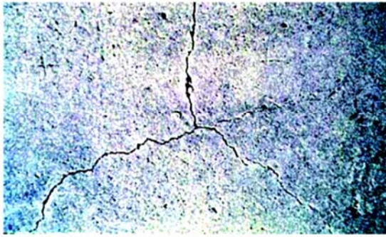
Figure 2-3: Shrinkage cracking (ACI 201.1R-08)
