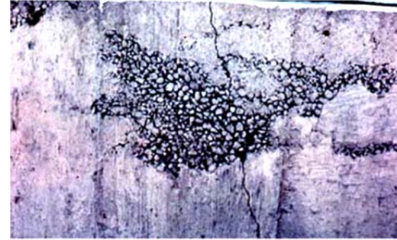
Figure 2-8: Concrete surface with honeycombing (ACI 201.1R-08)
