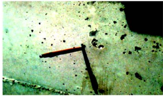
Figure 2-4: Surface air voids (also known bug holes, ACI 201.1R-08)
