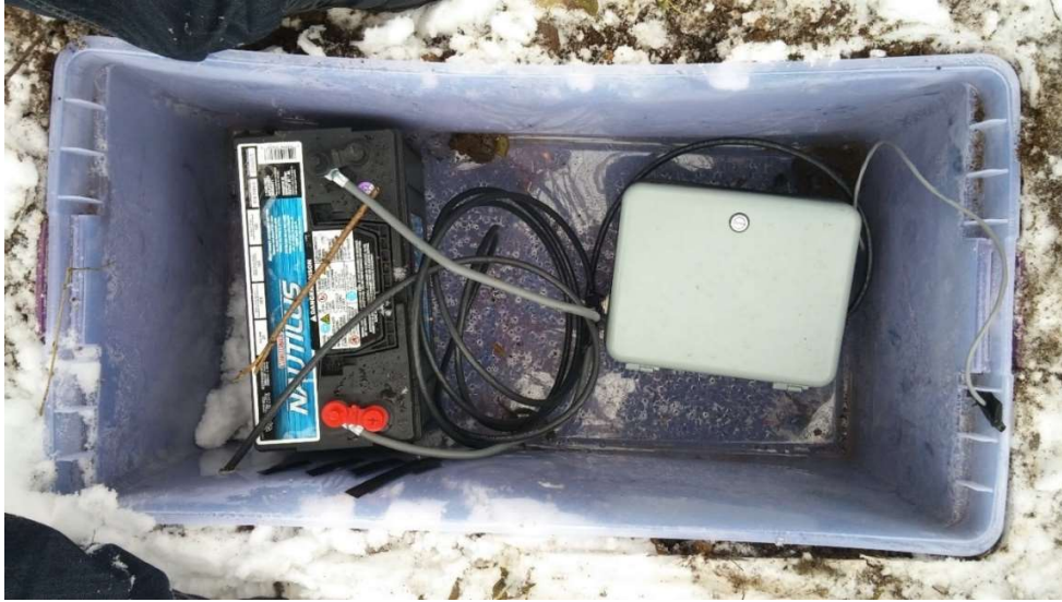
Figure 61: MAR and battery installed into the plastic container
