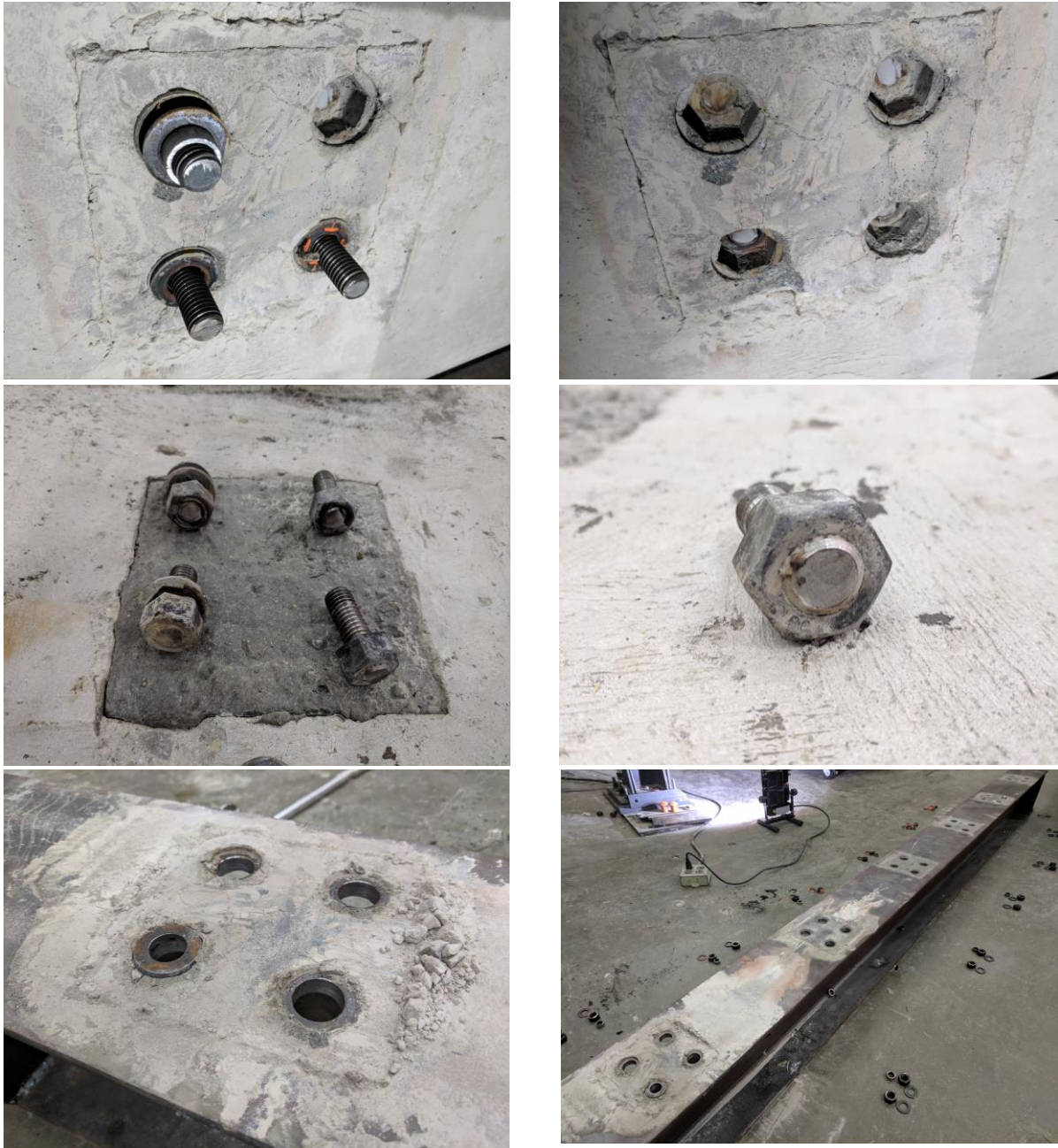
Figure 4-20: Failed bolt group of EB1 and concrete pulverization left on the top flange.
