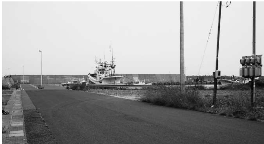
Figure 4.8 - The breakwater wall as seen from the northwestern entrance to the port.
